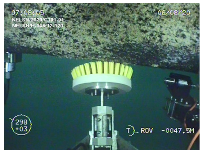
In-water photo of FMD system. UT FMD to left of screen at 6 o'clock position on member
